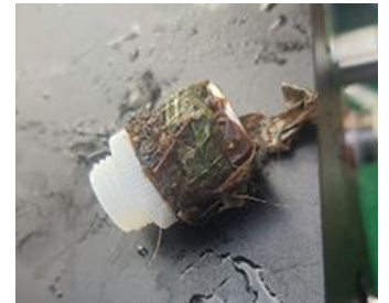
Clogged inline filter
